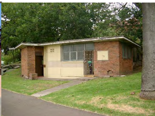
Condition 5 – Very Poor
