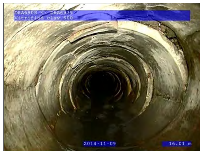
Condition 5 – Very Poor
