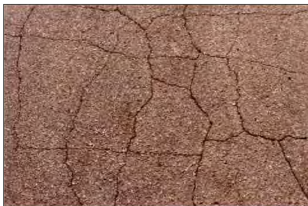
Condition 5 – Very Poor
